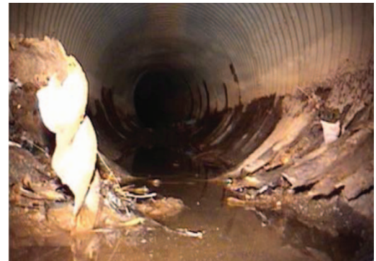
While we can't see the drainage pipes that support the most basic functioning of our city, we all rely on them to carry the overflow of water that rushes from our streets, parking lots, yards and farms during storms.
